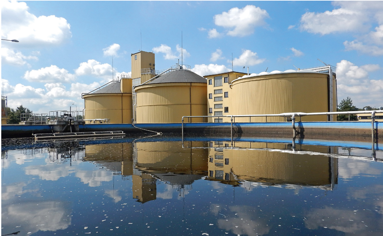
Photo 2. Digesters (2x5500 m 3 )
