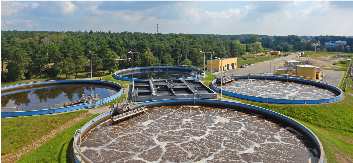
Photo 1. Modernised biological part of the plant - C-TECH Technology sequenced chamber
