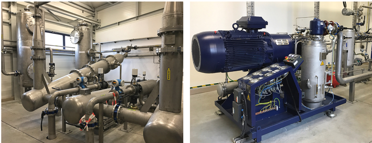
Photo 4. Biogas Purification System absorbing carbon dioxide
